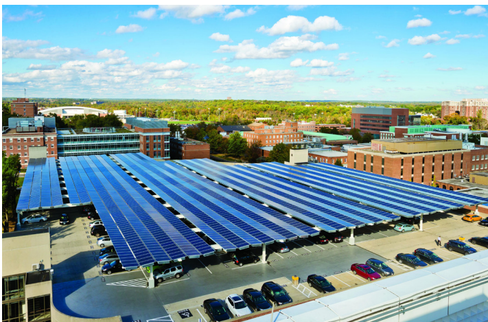
Use of Photovoltaics (Example: Regents Garage PV Panels)
