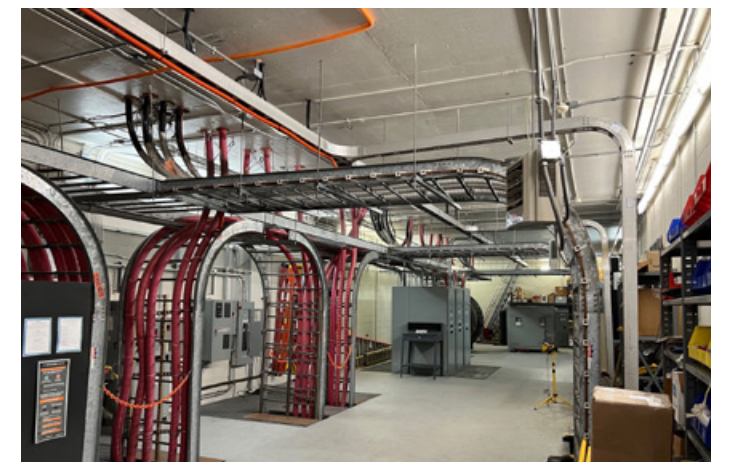
The Mowatt Substation recently received upgrades but may be reaching capacity
