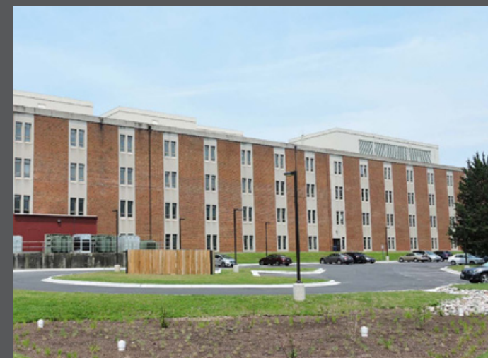
Partial demolition of A.V. Williams after programs are relocated to A.I. and Machine Learning building provides space for Paint Branch Green
