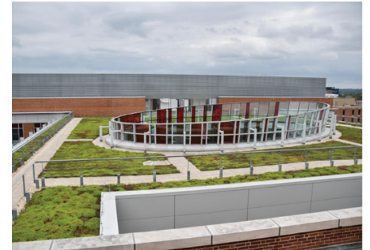
Existing Stormwater Management Practice: Rainwater Harvesting (Example: Physical Sciences Complex Green Roof)
